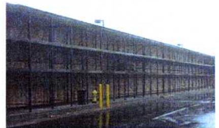
Pallet rack interior fence
