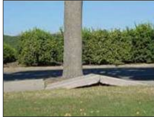
Subsurface tree roots can lift concrete sidewalk slabs, causing the surface to become uneven.
