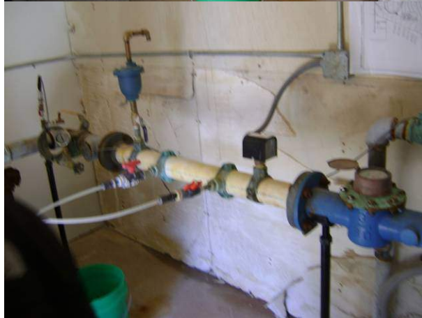
Chemical injection pumps
