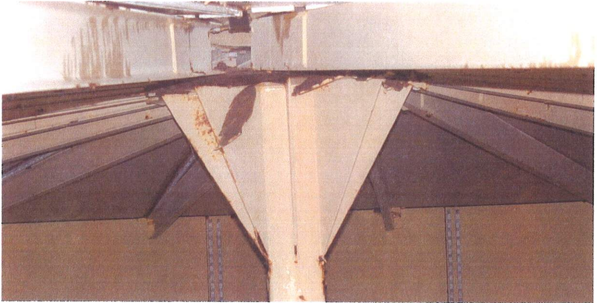
Corrosion at Center Column/Roof Rafters
