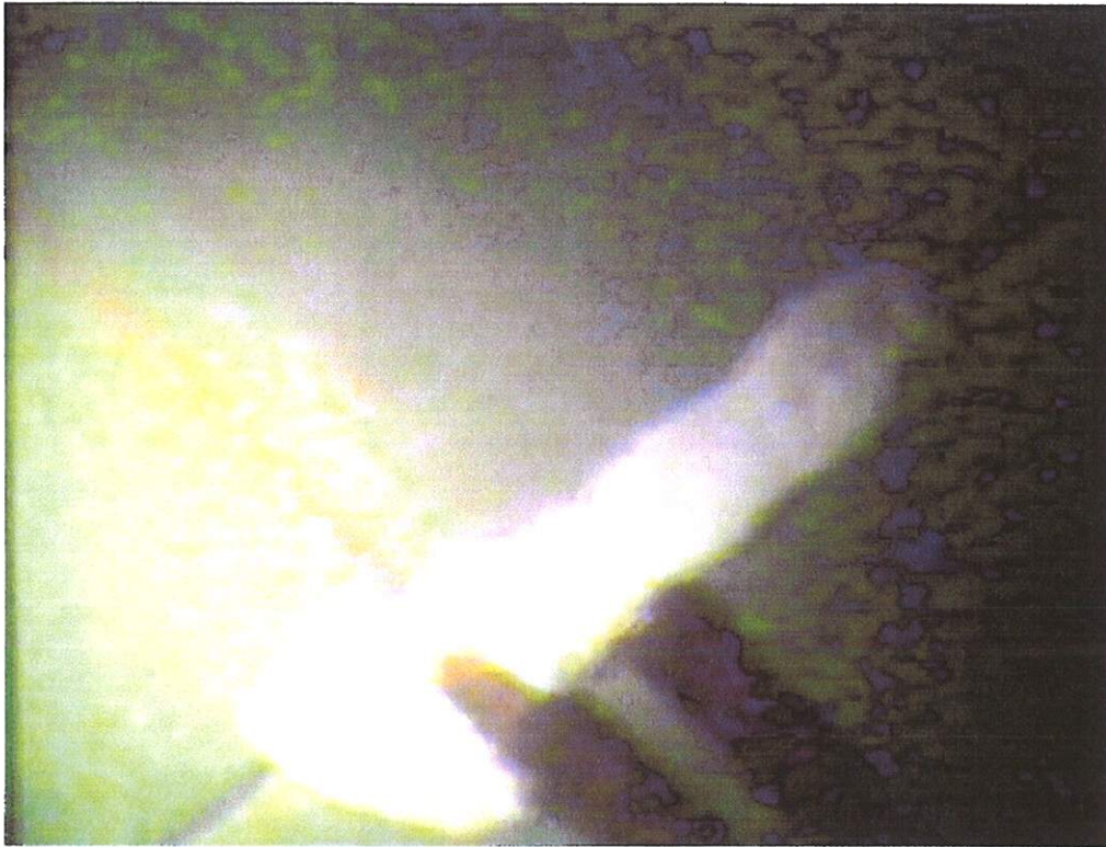
Previous Epoxy Repair
