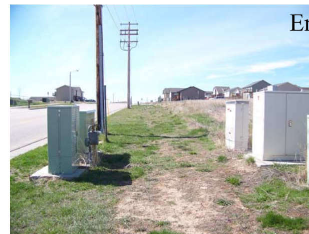
View to south, path between utility boxes.
