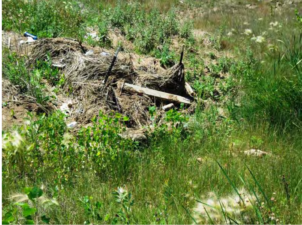
Element 5: Inlet End of Pipe in Pond 101 is Covered with Debris
