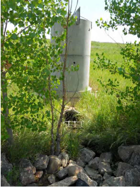
Detention Pond 100: Riser
