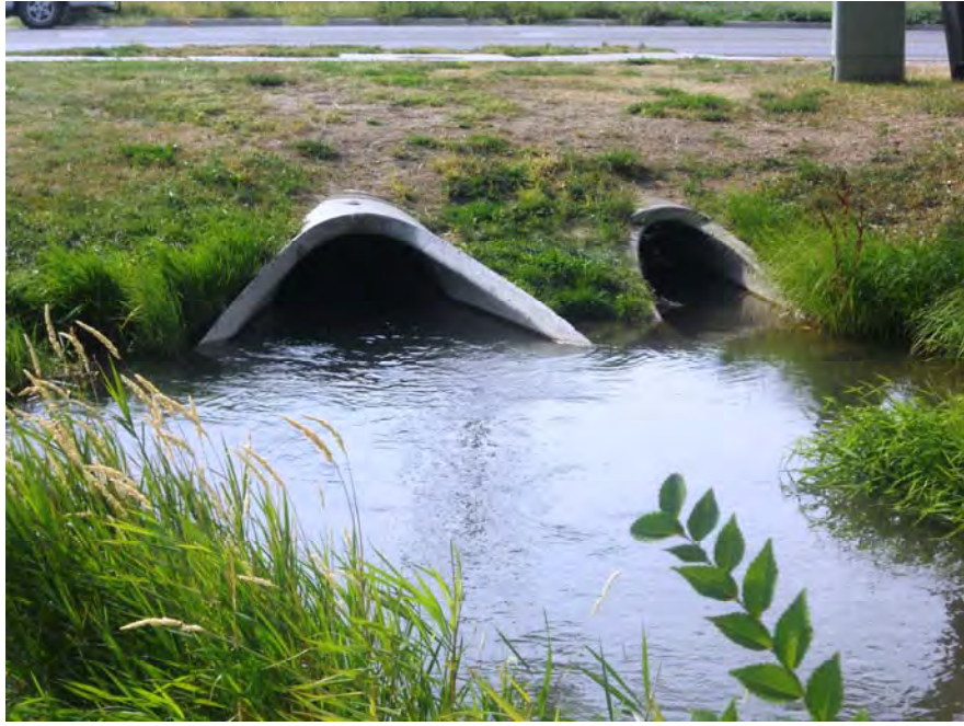
H1: Hawthorne Ditch at Covington Street Discharge (irrigation on left, storm on right)
