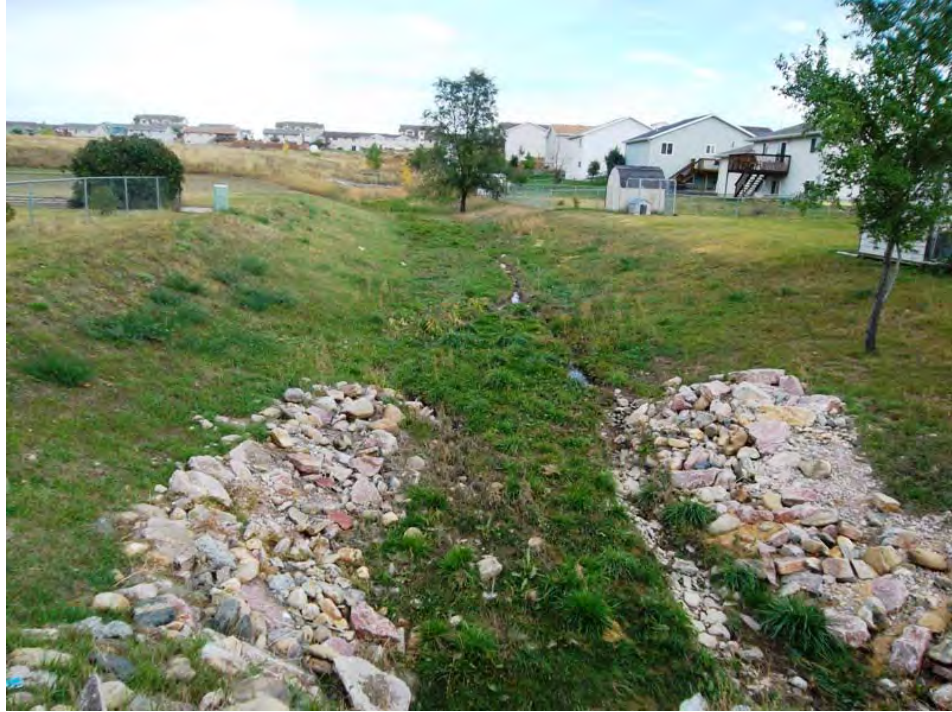
Element 10: Looking Upstream from Avenue A, Element 9 Outlet is Indicated by Red Box
