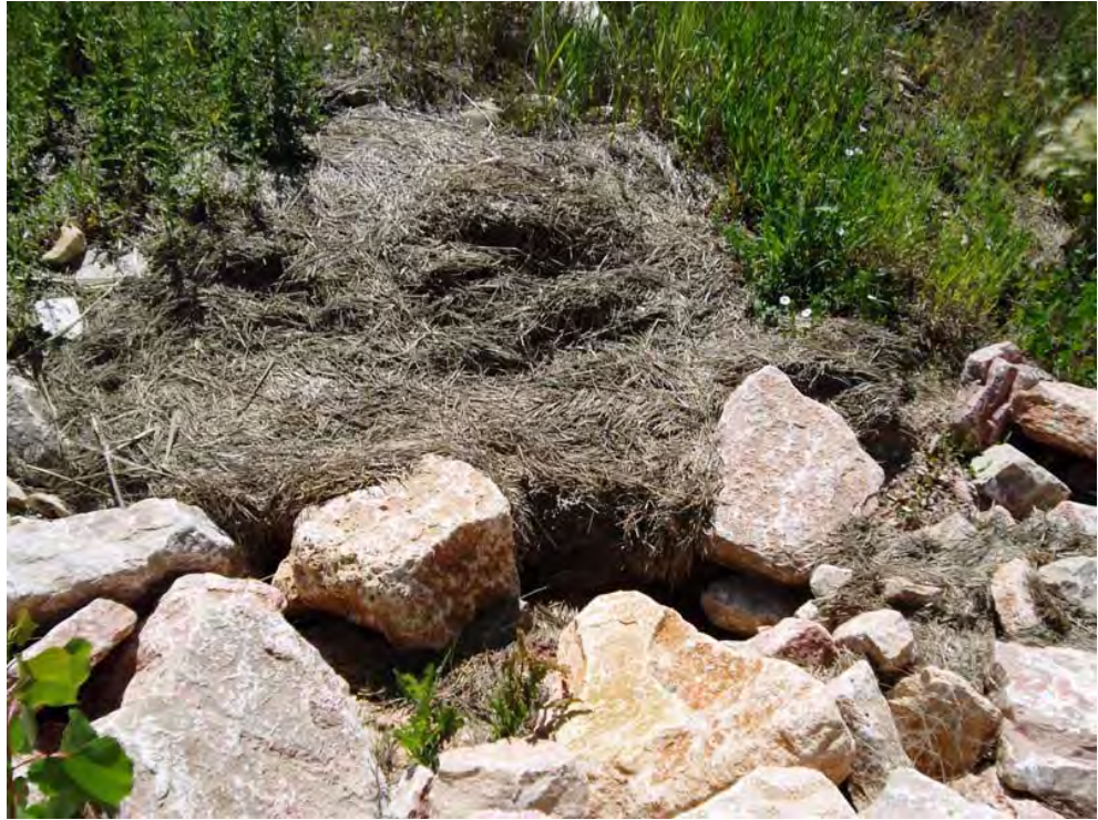
Detention Pond 104: Inlet End of Pipe Covered with Debris
