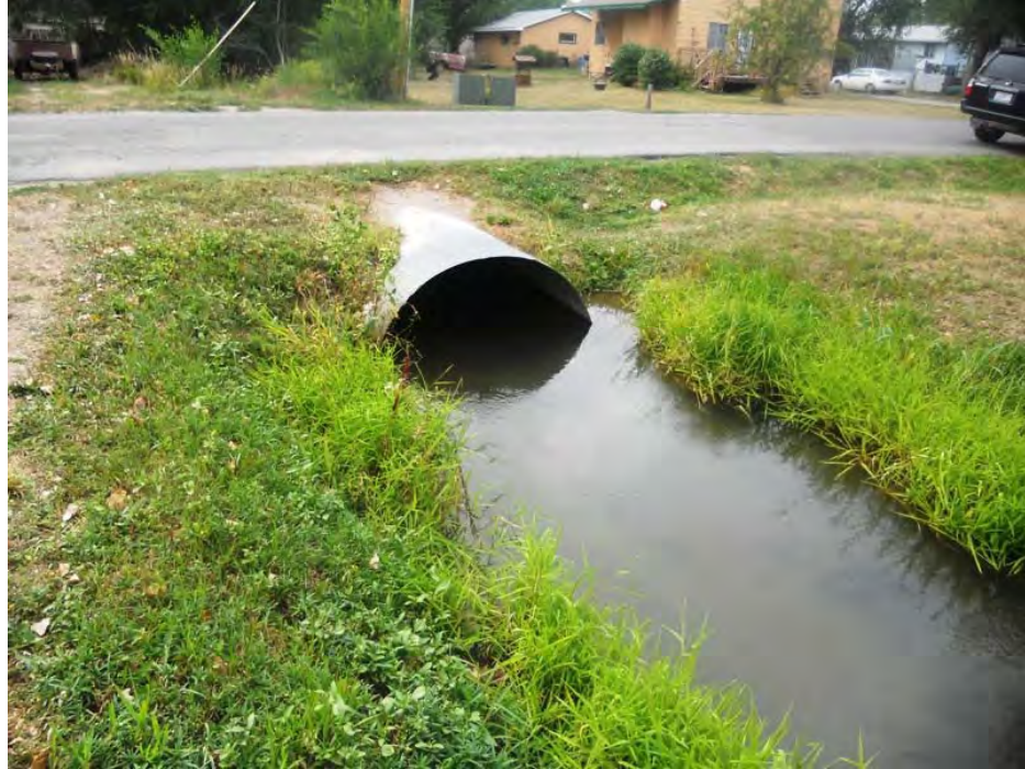
H5: Hawthorne Ditch at Plateau Lane (outlet end is shown)
