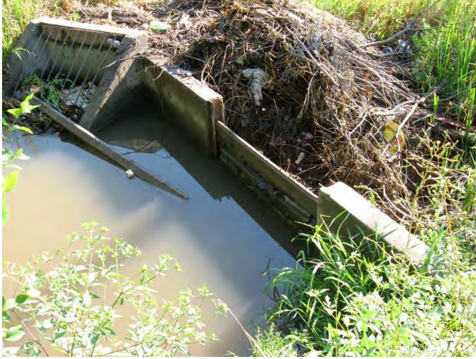
H13: Hawthorne Ditch Siphon Inlet and Waste Gate (West of the Albert Street box culvert outlet)
