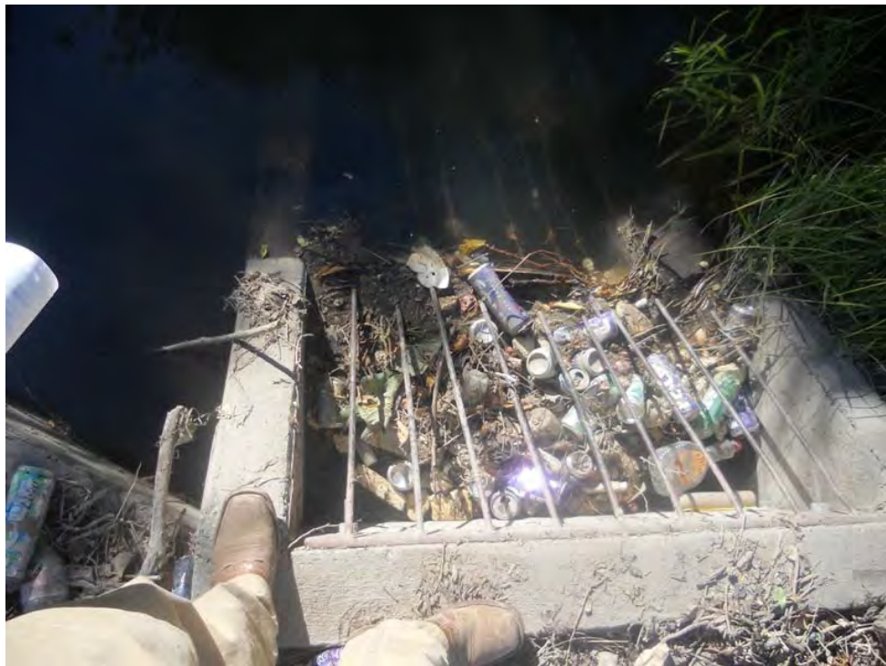
H14: Hawthorne Ditch Siphon Inlet (Top View of Siphon Trash Rack)
