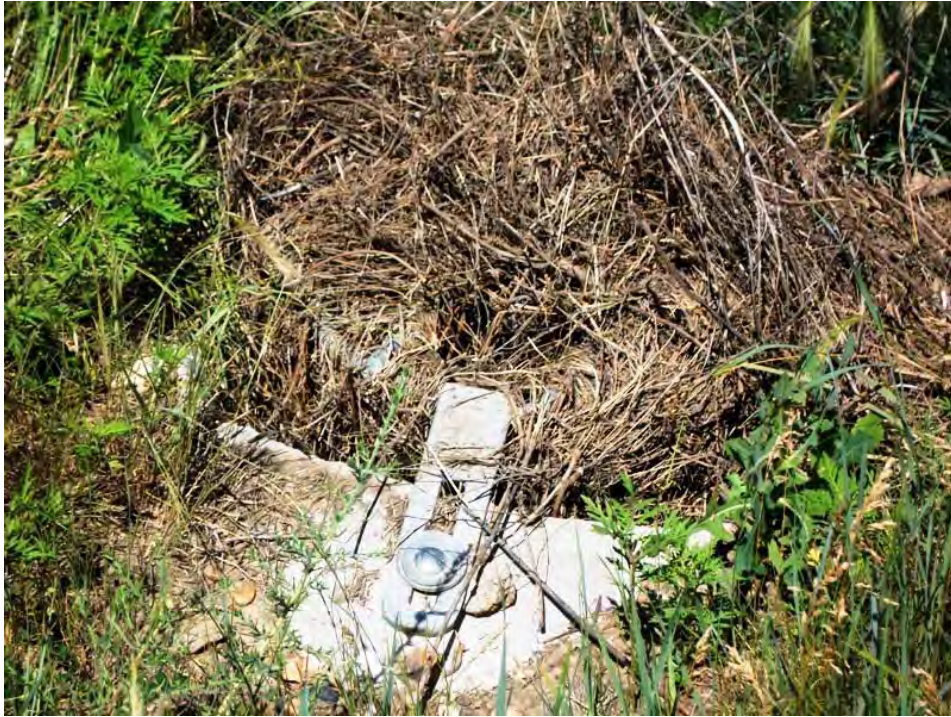
Element 1: Low Flow Pipe Inlet located in Detention Pond 103
