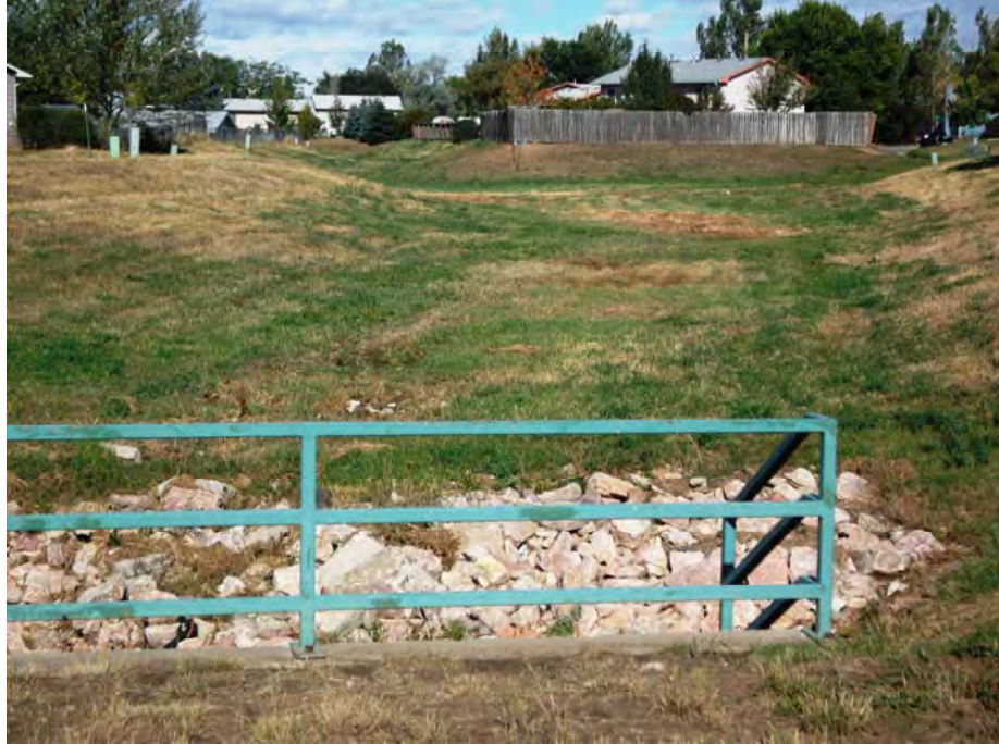
Element 12: Looking Upstream from Twilight Drive, Also Shows Element 7 Channel Entering on Right & Element 11 Channel Beyond
