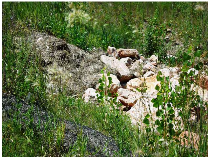
Element 3: Inlet End of Pipe Covered with Debris, Located in Pond 104
