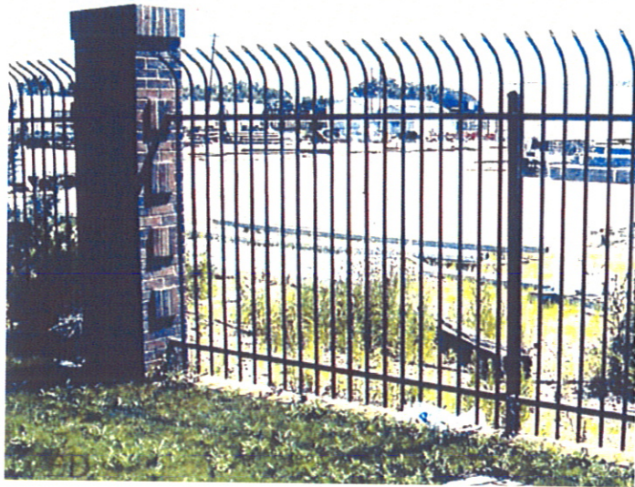
5th Street Substation, Typical Corner/Gate Post
