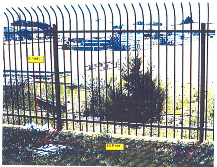
5th Street Substation, Typical Fence Section
