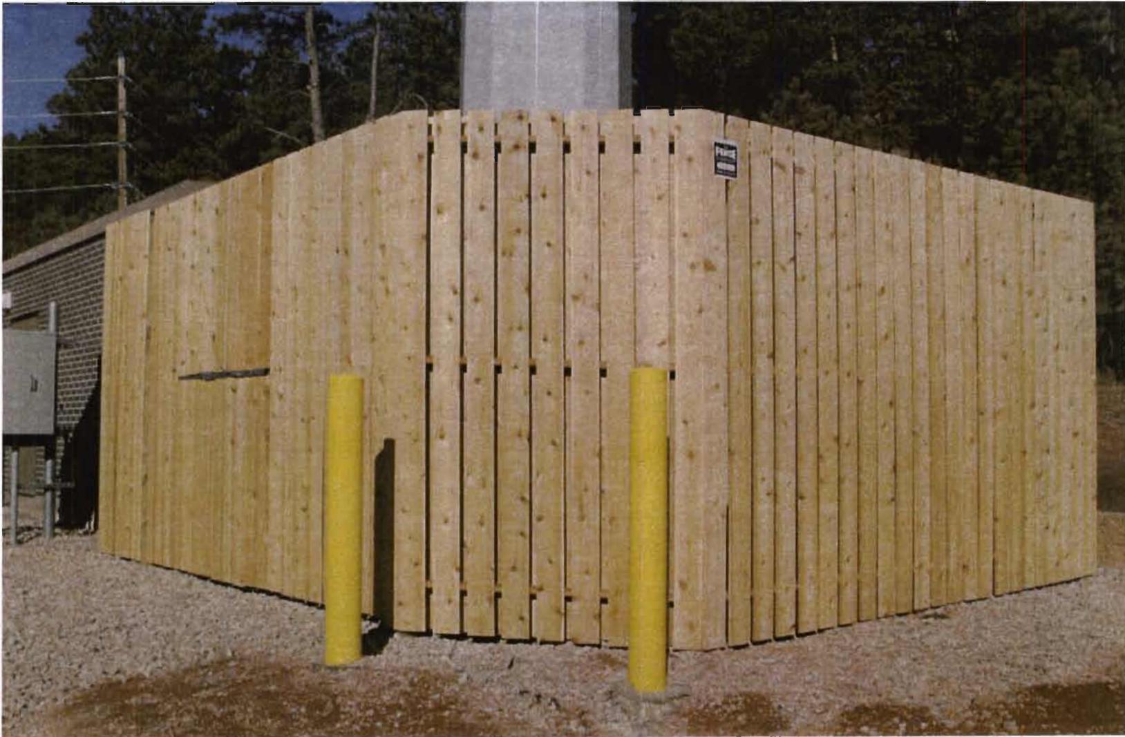
The wooden fence that encloses the base of the Verizon Wireless flag pole.
