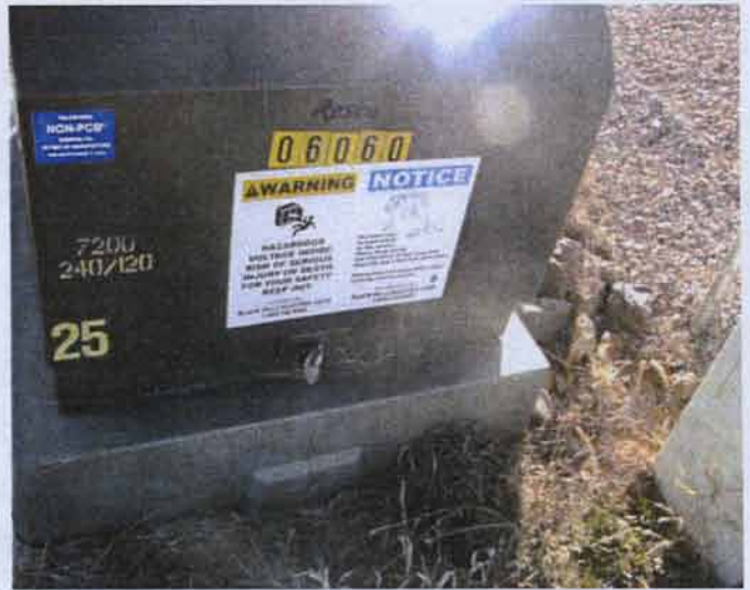
POWER (TELCO CLOSE)
