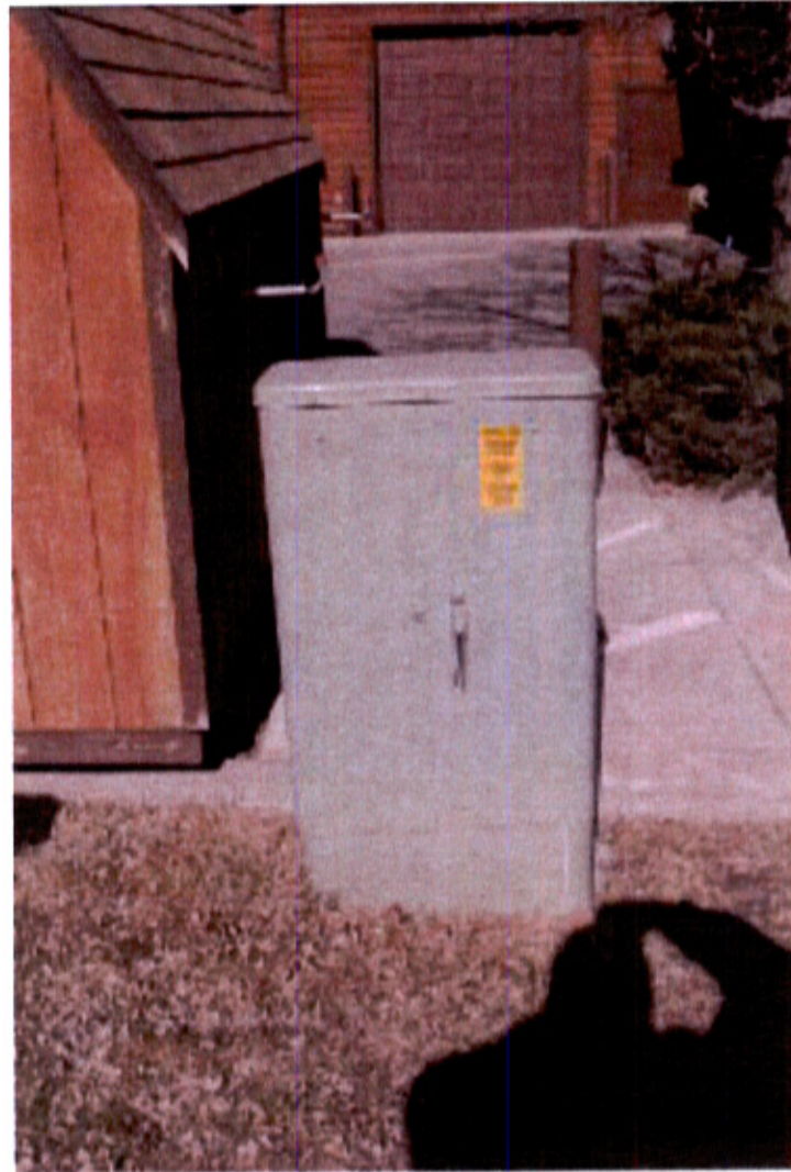
A telco or fiber pedestal located on the south side of the property.
