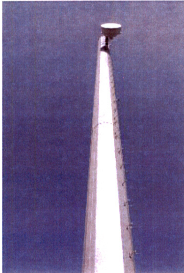
View looking up at the south face of the Golden West monopole.
