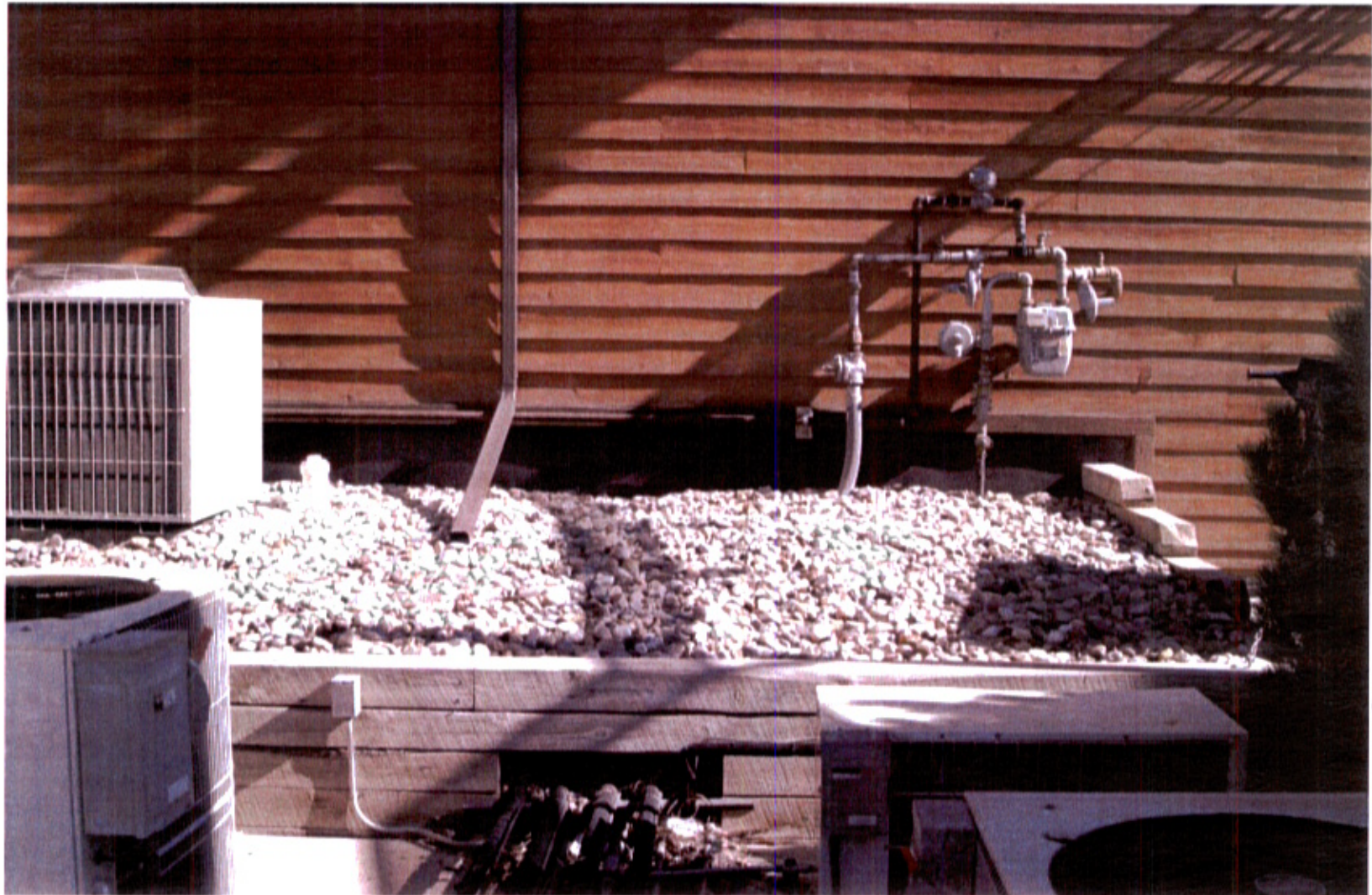
If radio equipment needs to be located outside, this location on the west side of the building might be just large enough to hold our equipment. However, please note the air conditioning lines running under that area.
