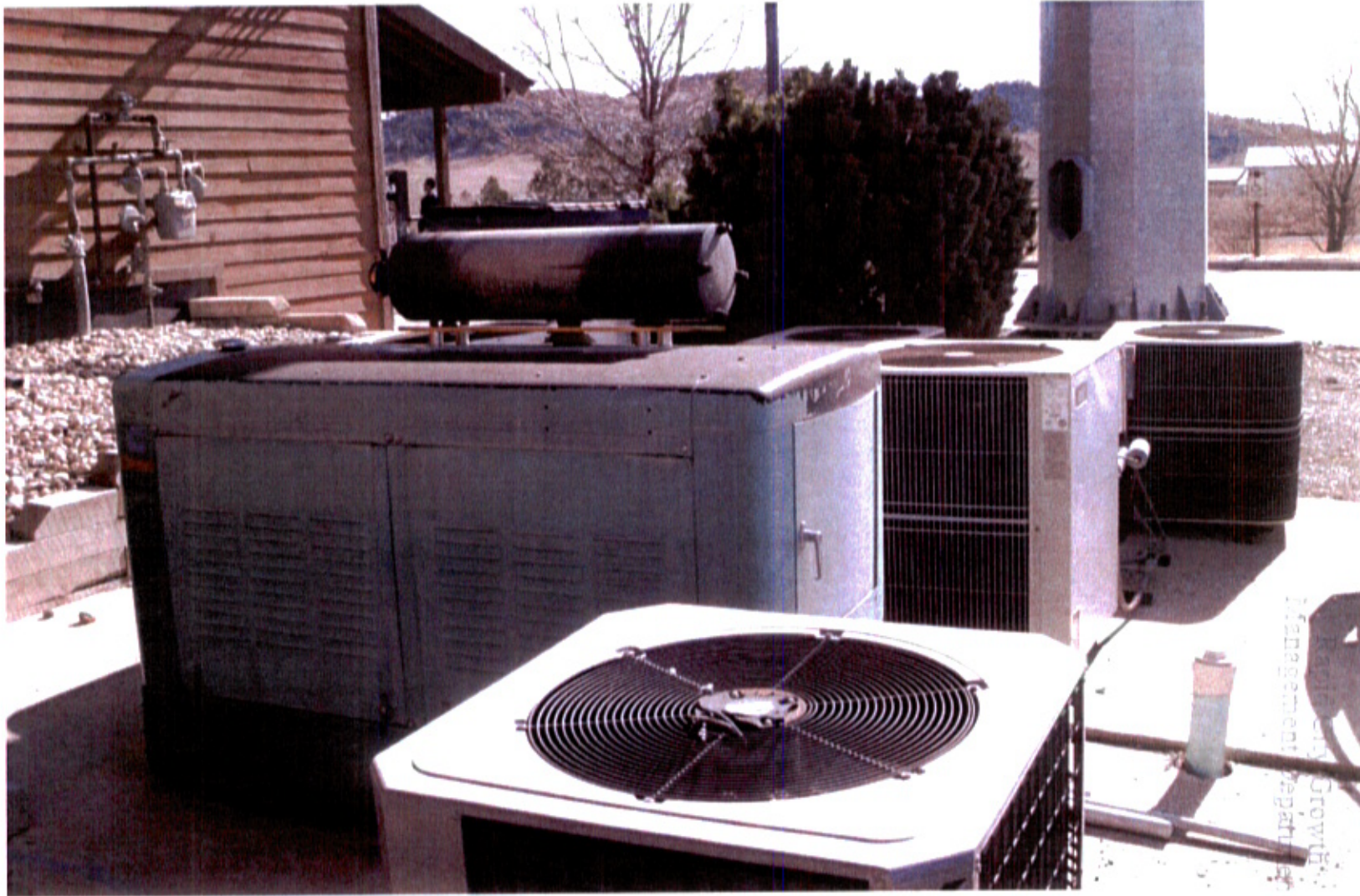
A view of the generator and many air conditioning units near the base of the monopole.
