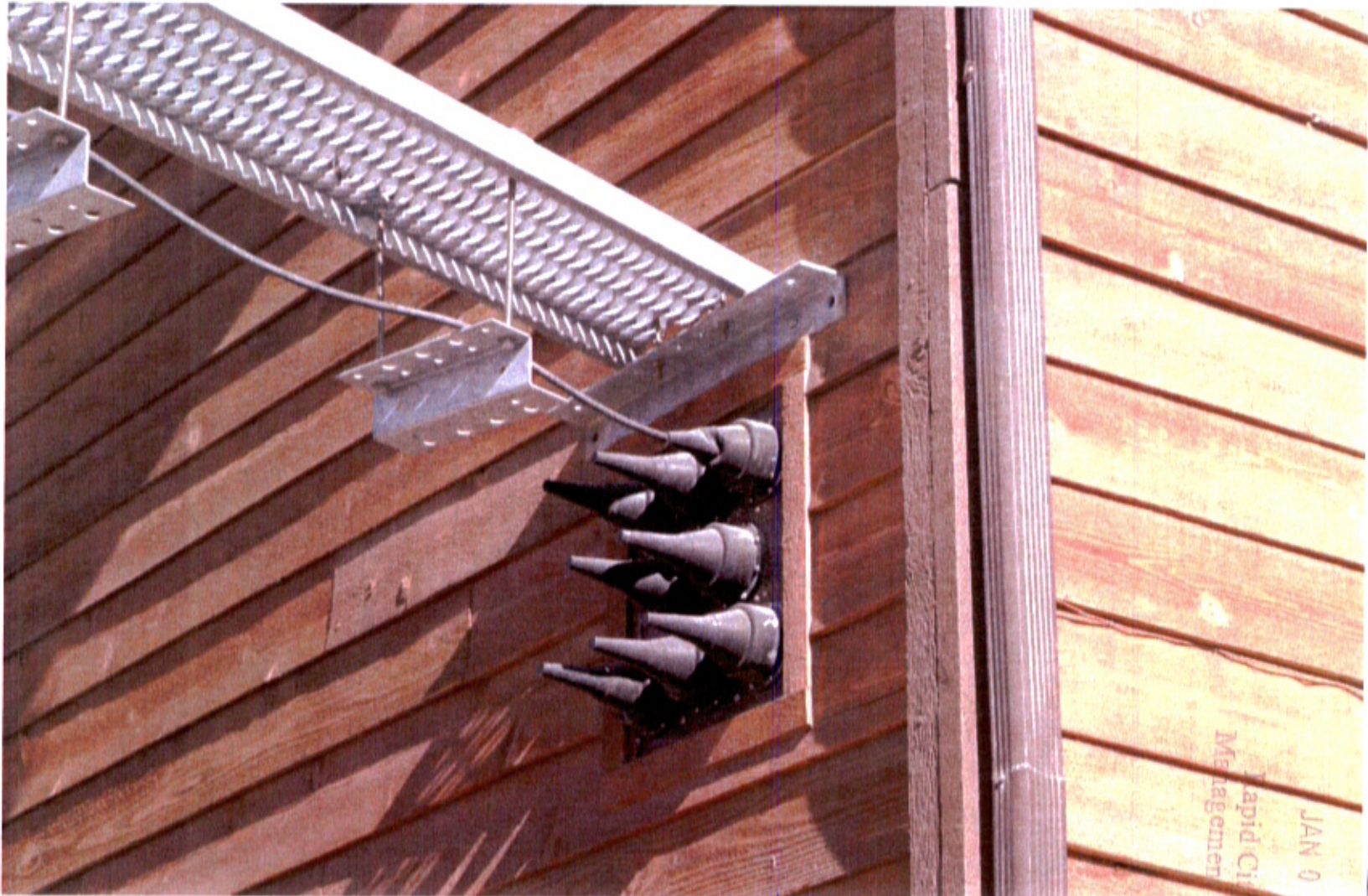
Existing entry port on the side of the Golden West building. This would indicate to me that there is probably space inside the building for our radio equipment.
