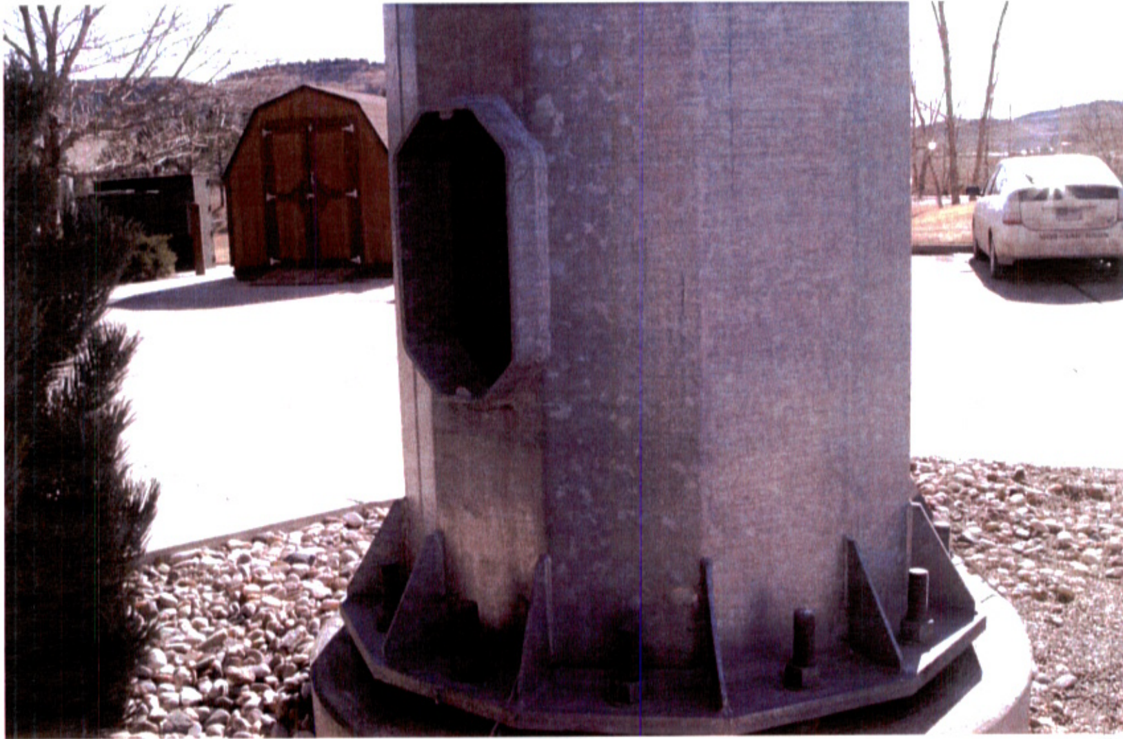
Available exit port on the east face of the monopole.
