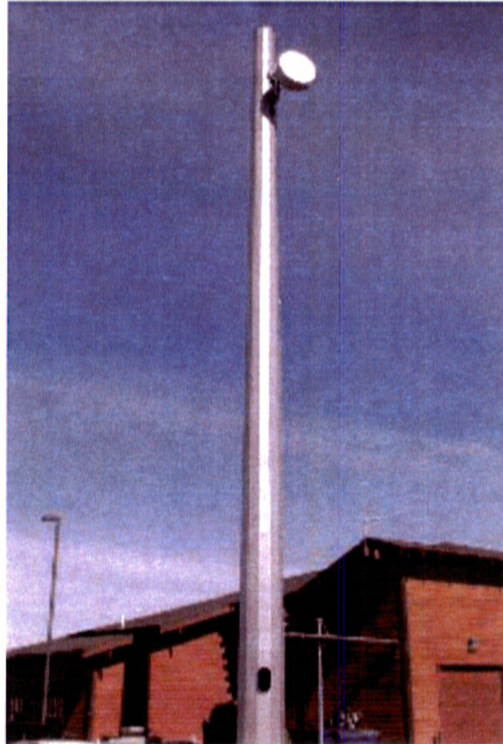
Looking up at the southwest face of the existing monopole. Please note the small 3' point-to-point dish at the top.
