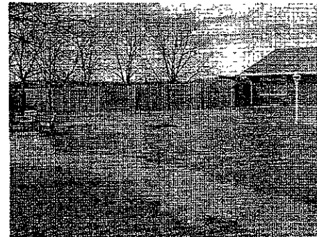
EXISTING FENCED-IN YARD BETWEEN WEST WING AND SOUTHWEST WING - EXISTING FENCE, SIDEWALK, AND LIGHT POST TO BE REMOVED - EXISTING FURNITURE TO BE RETURNED TO OWNER
