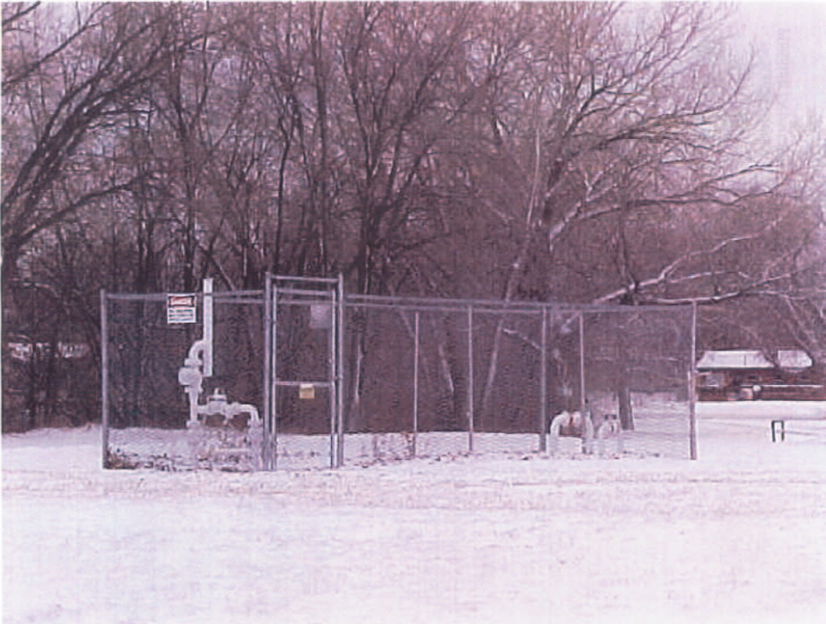
Similar utility substation
