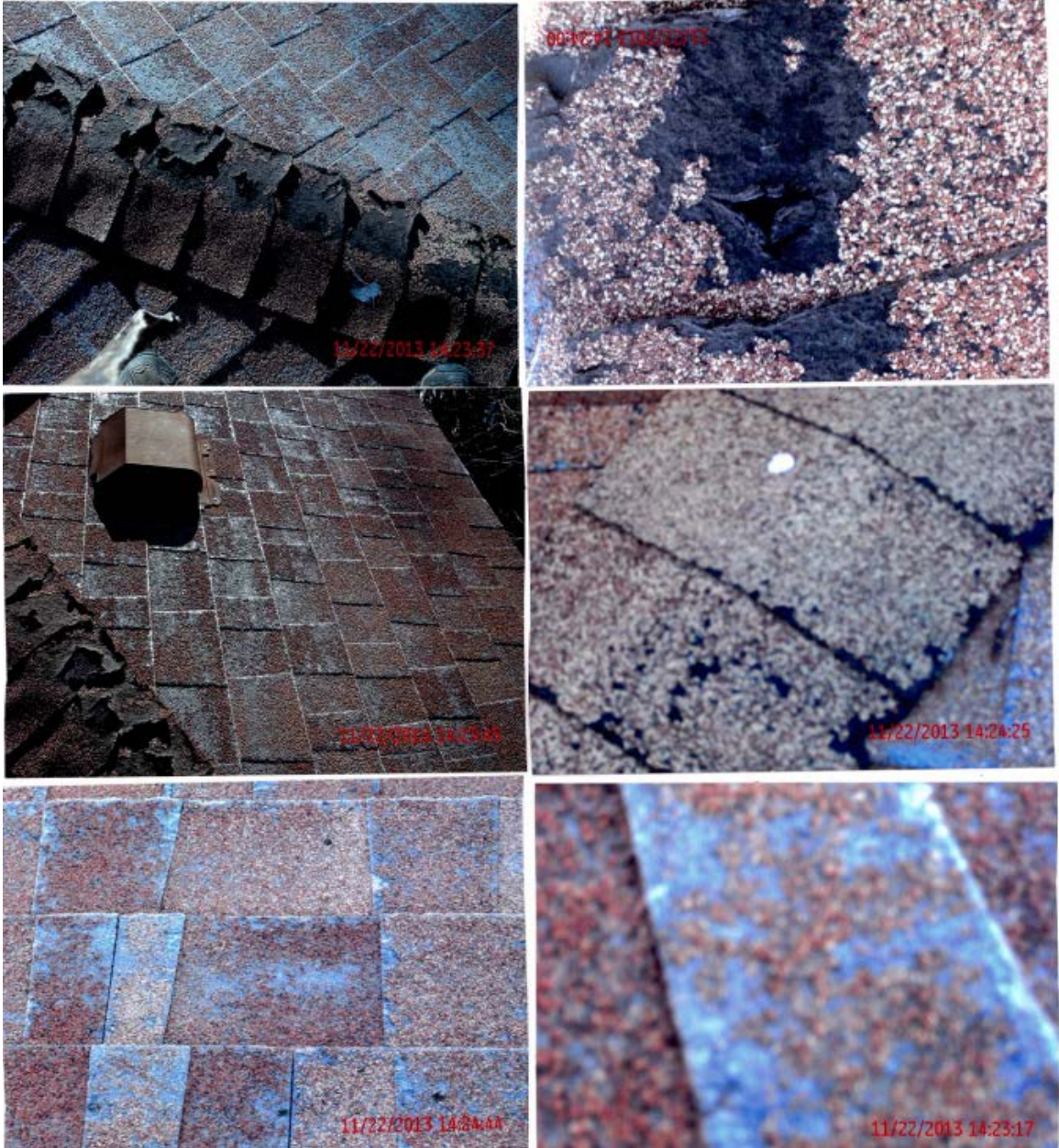
Figure 4: Existing Damage to Roof at 1116 South Street
