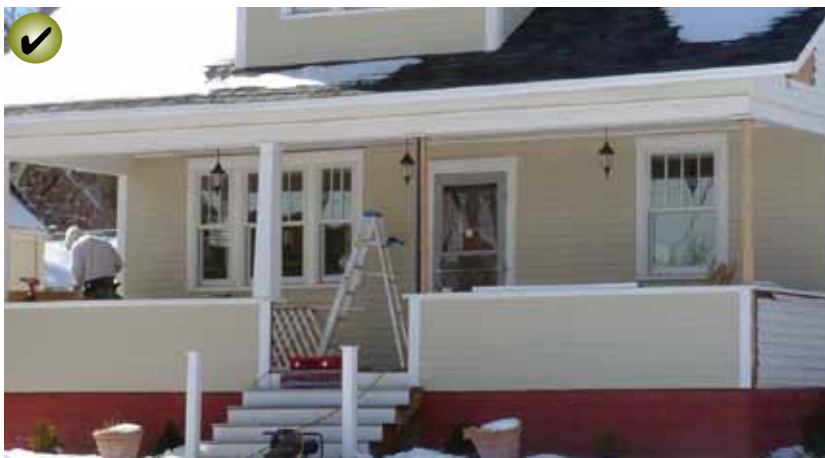
Repair those elements of a porch that are deteriorated.
