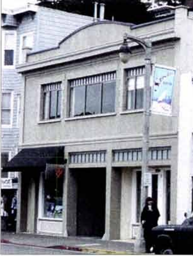
A parapet wall (An upward extension of a building wall above the roofline) should not be altered, especially those on primary elevations or highly visible facades.
