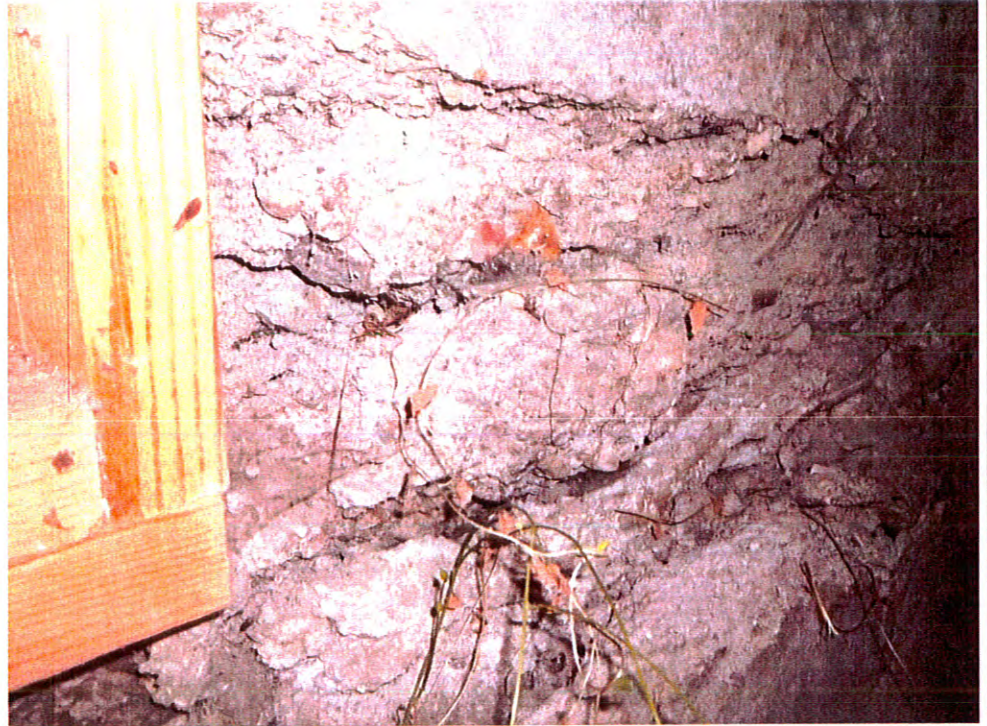
Bind weed growing through the wall on the interior of the basement
