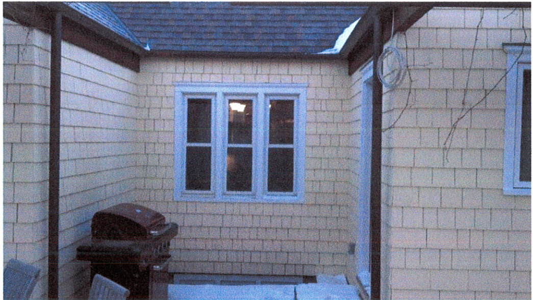
Rear of house (faces west). Windows to be replaced with matching casement (wood).
