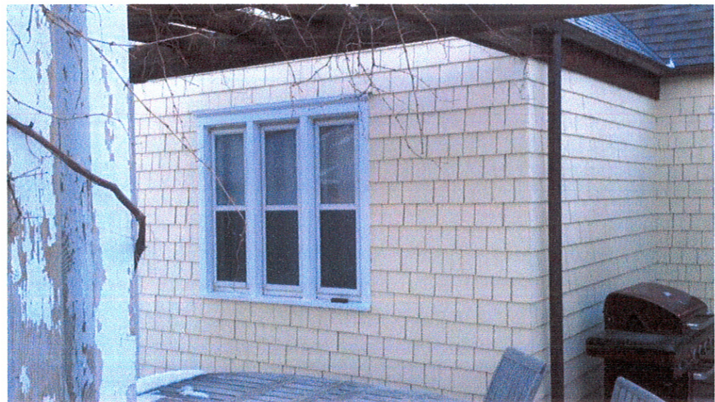
Rear of house (faces west) – bedroom windows to be replaced.
