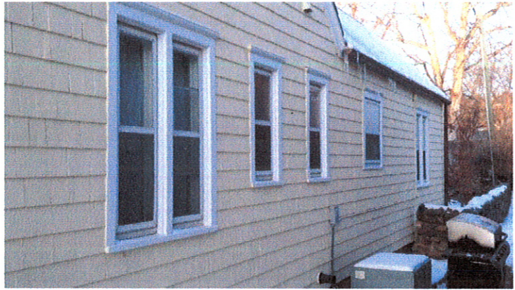
View of north side of house looking west. From east to west: set of original bedroom windows, original bathroom windows; non-original bathroom window, set of bedroom windows.
