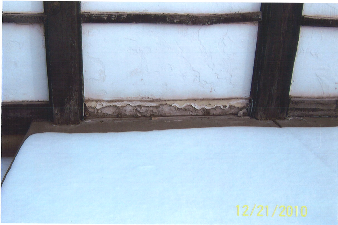
Exterior building damage
