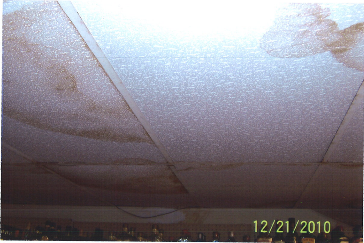
Interior ceiling damage
