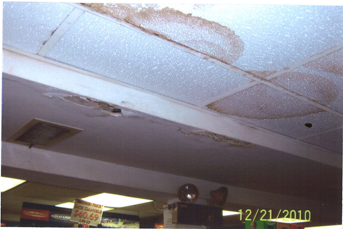
Interior ceiling damage
