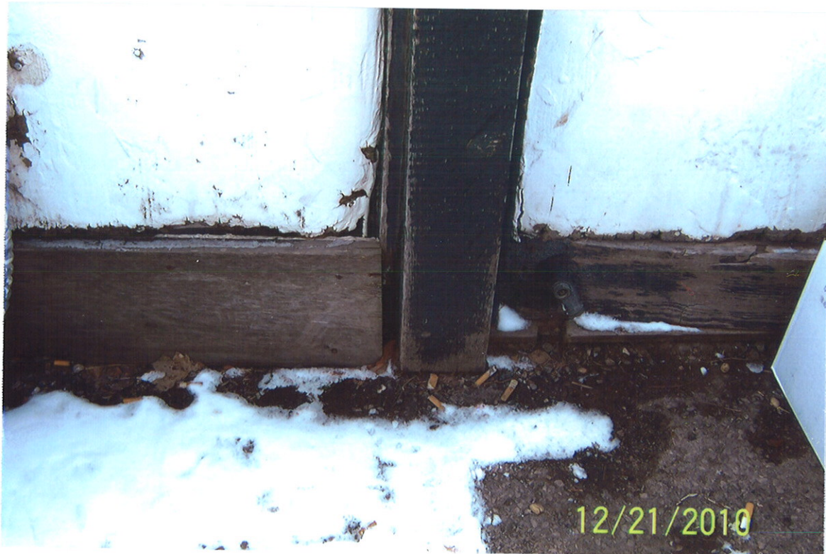
Exterior building damage
