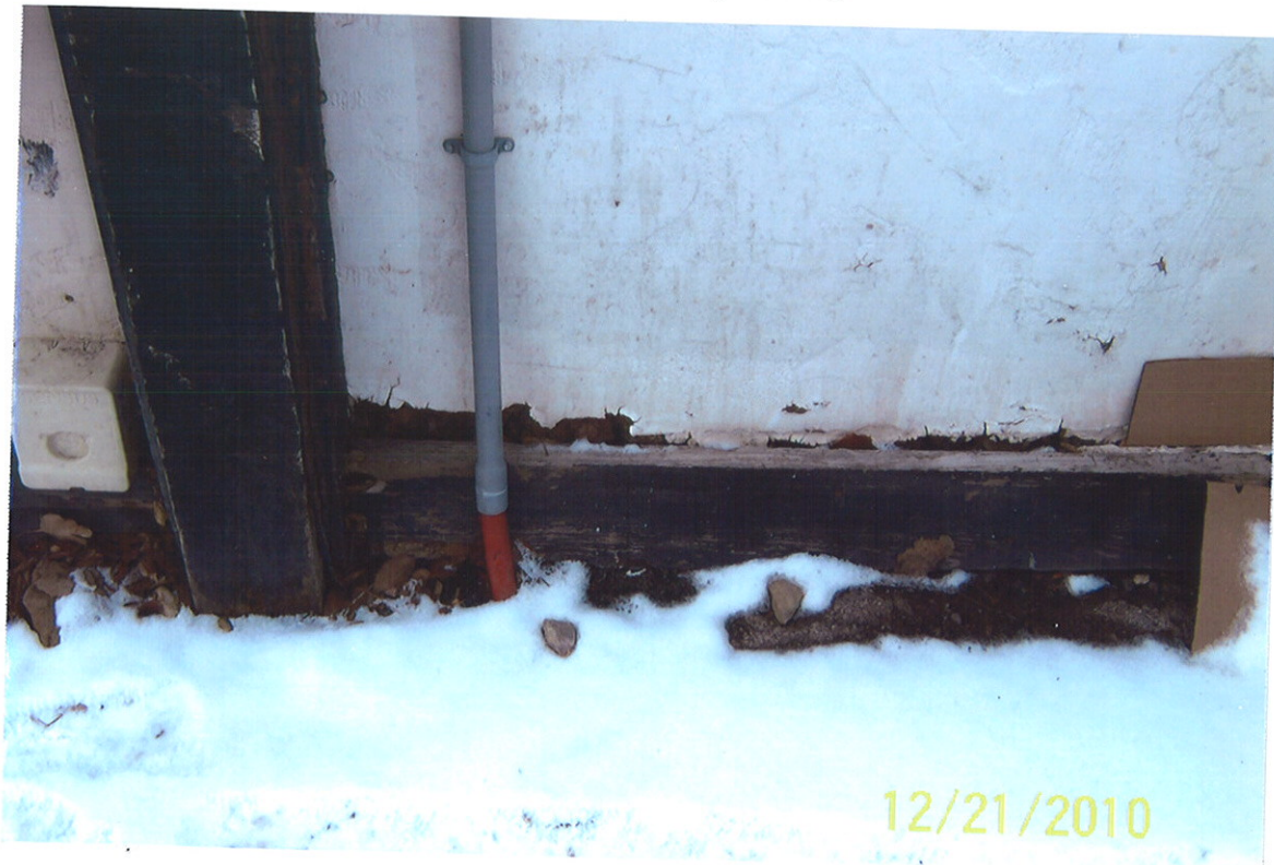
Exterior building damage
