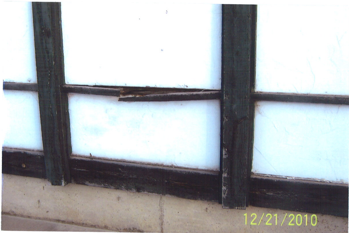
Exterior building damage
