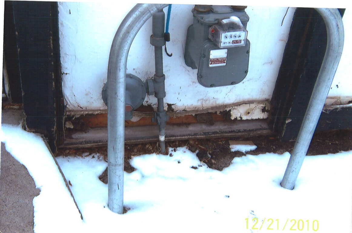
Exterior building damage
