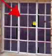
Window 36 Mechanical Room
