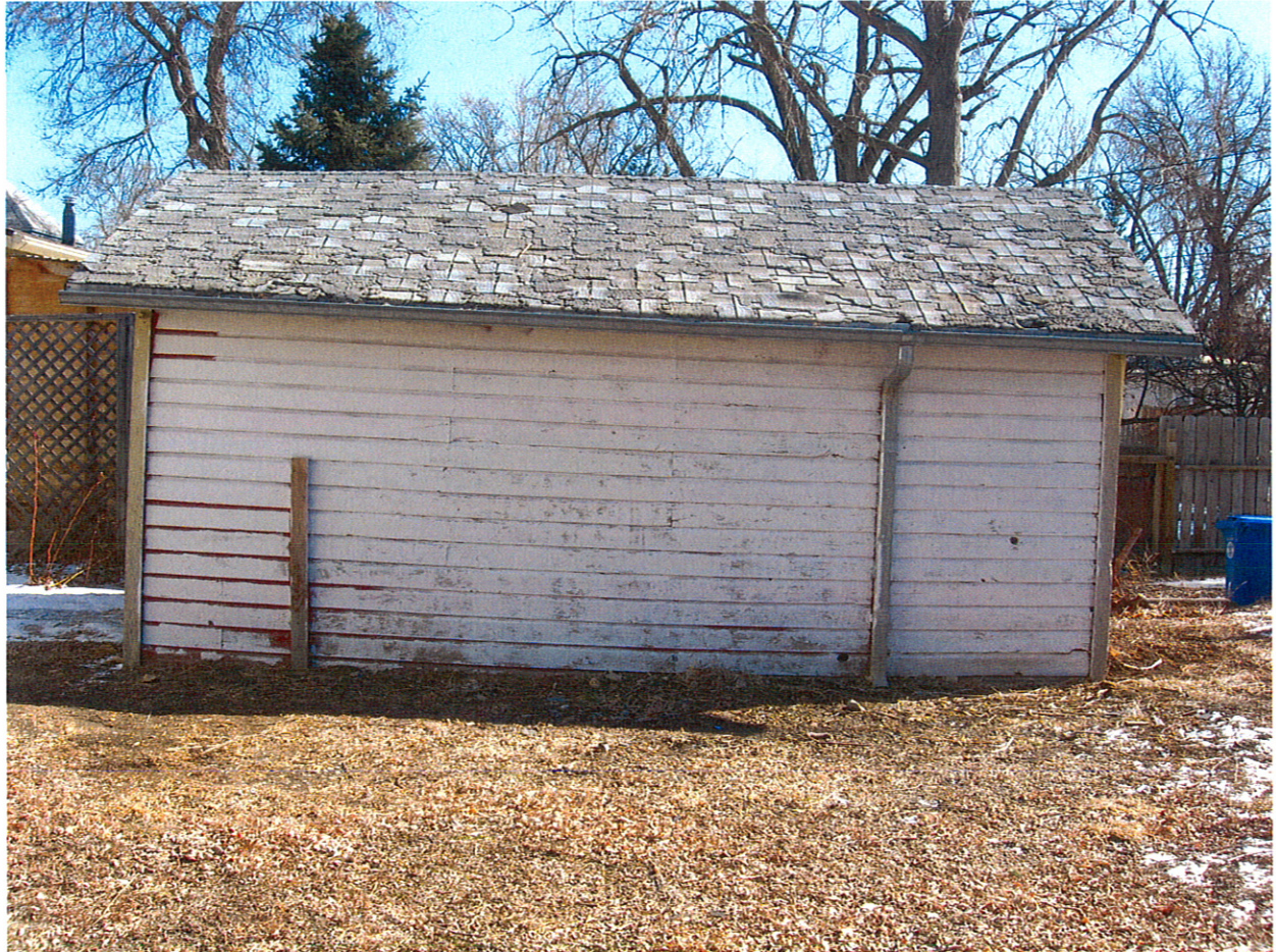
Photo 2- West wall exterior – note bow in roofline
