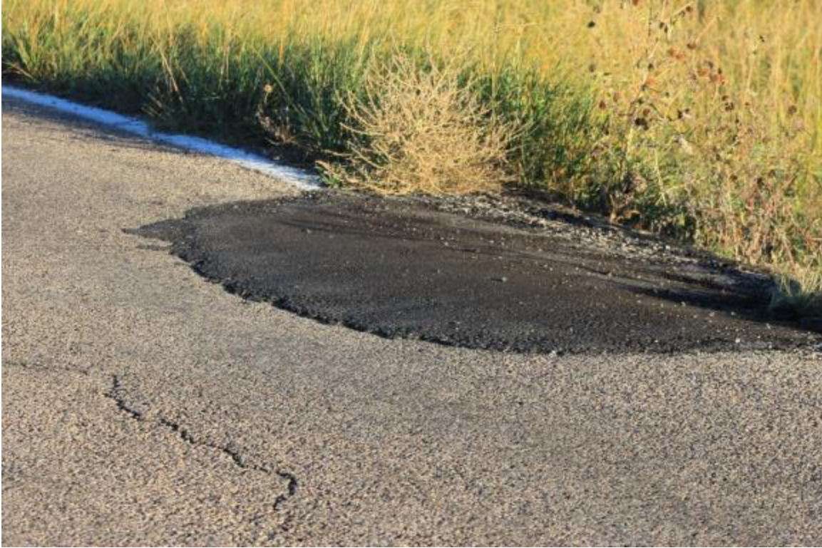
Patchwork on culvert with a dip all the way across.
