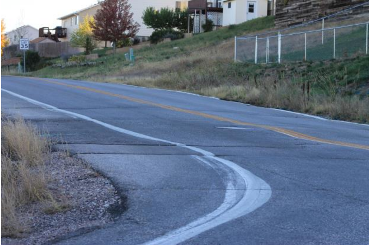
This patch has been done and redone at least twice if not 3 times.
