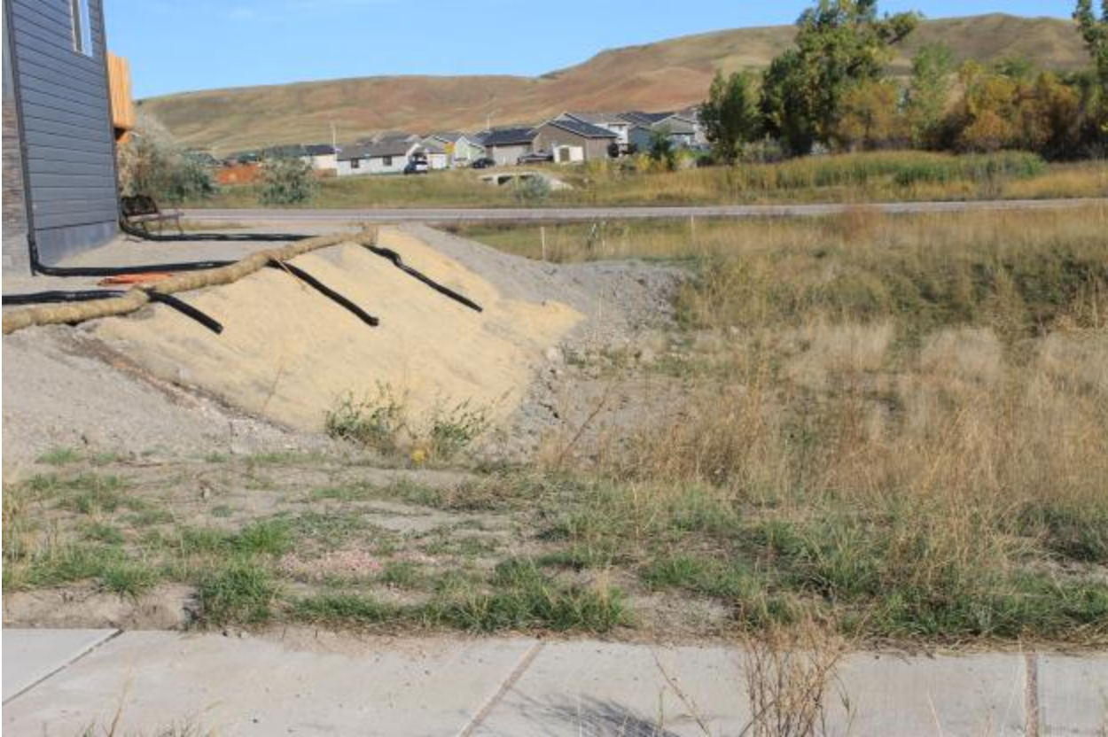
House built into the sidewall of a detention pond in phase 3 of Freeland Meadows subdivision.
