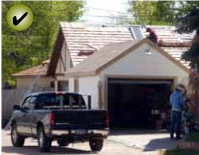
New or replacement roof materials should convey a scale and texture similar to those used traditionally.
