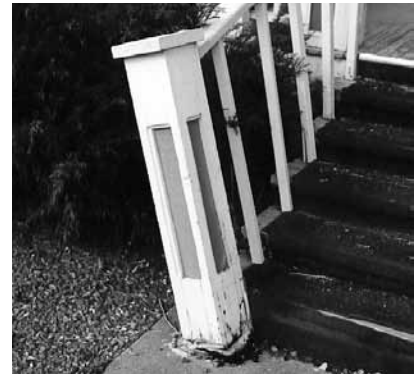
Before: A deteriorated post should be repaired not replaced when feasible.
