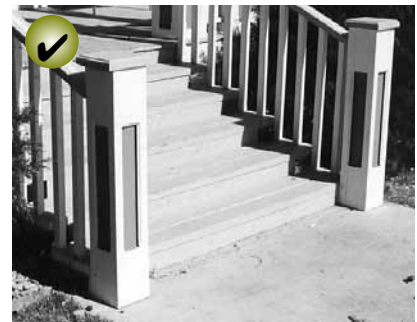
After: The base of the post has been repaired. This is an appropriate approach.
