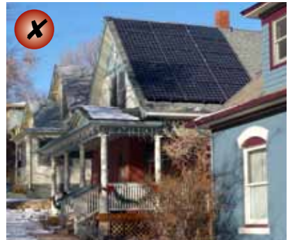
These collectors are inappropriate as they contrast too strongly with and overwhelm the character of the historic roof. They are also not sufficiently set back from the primary facade.
