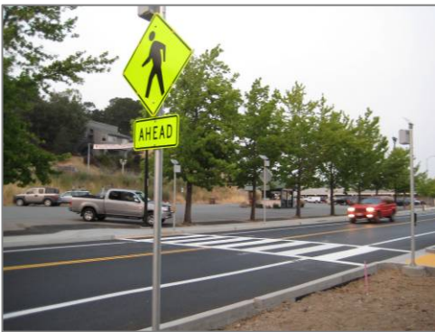
Figure 48. Example high-visibility crosswalk with fresh paint and a warning sign with flashing lights.
