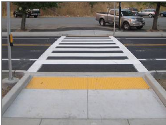
Figure 40. High-visibility crosswalk near a school in Fairfax, CA
