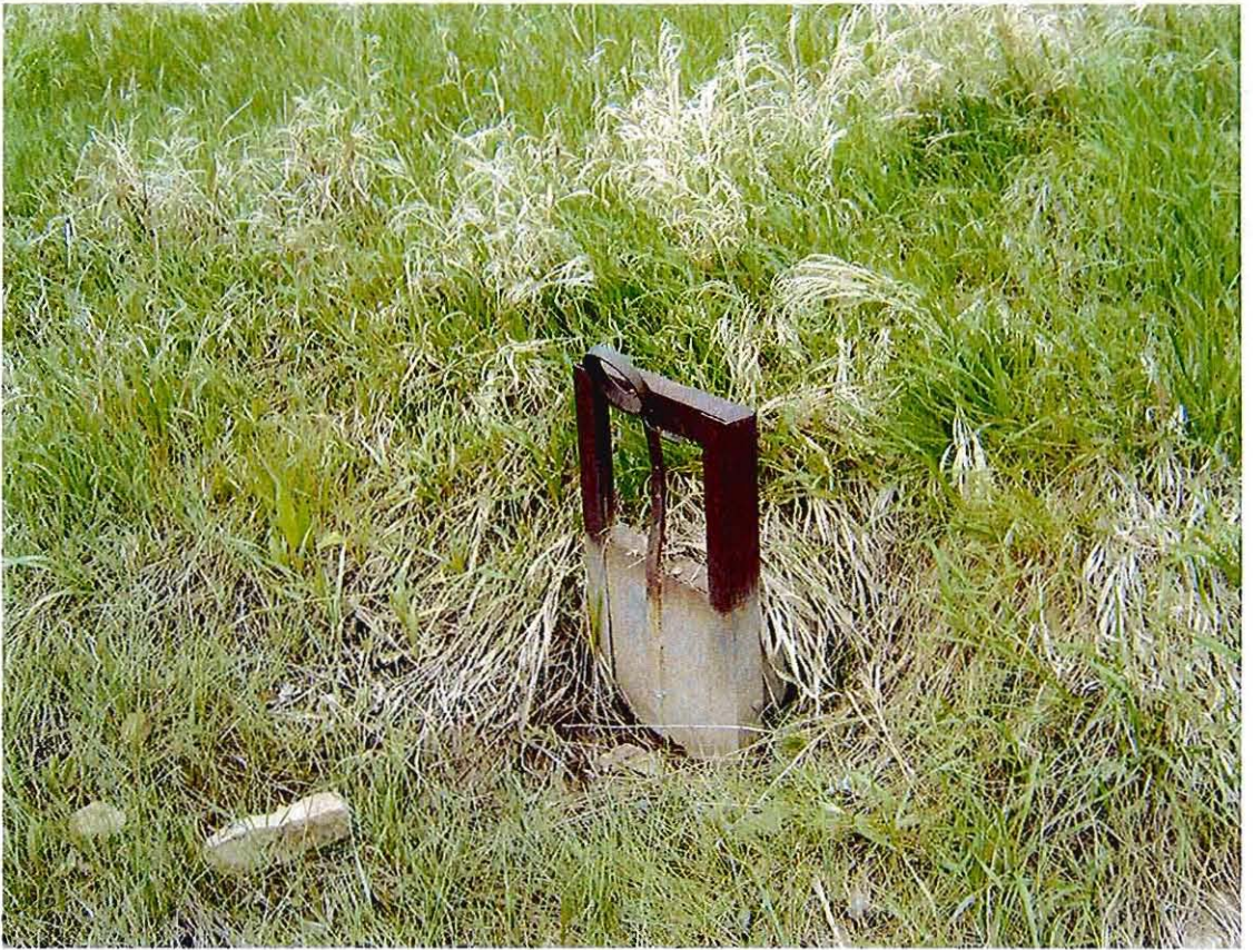
METER POND OUTLET GATE (CLOSED)
