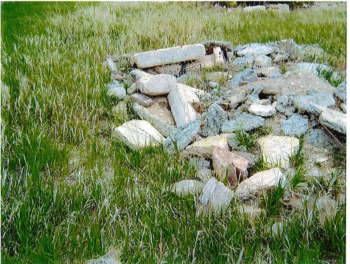
12" PIPE INLET AREA (PIPE NOT VISIBLE, MAY BE OBSTRUCTED)
