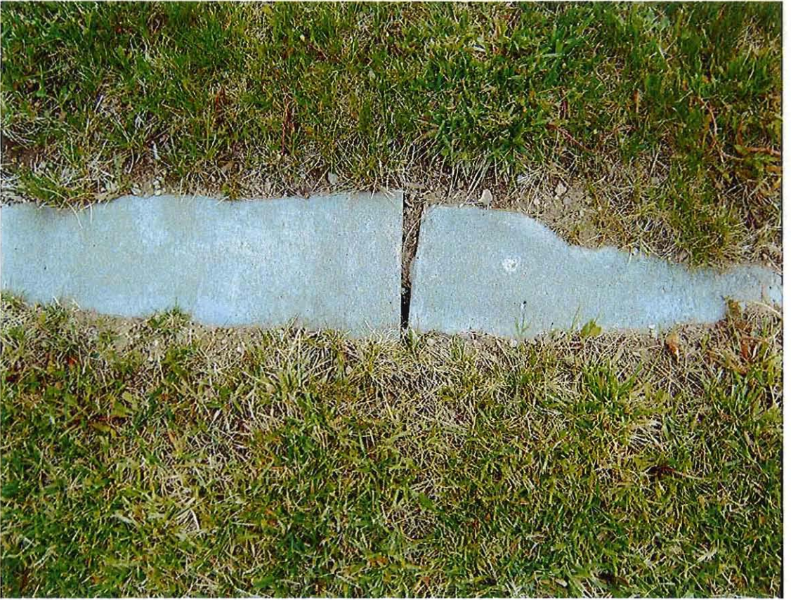
OPEN JOINT IN 12" PIPE 1317 HERMAN STREET
