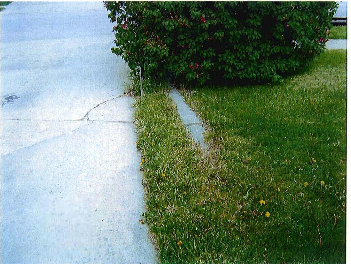
EXPOSED 12" PIPE AT 1317 HERMAN STREET
