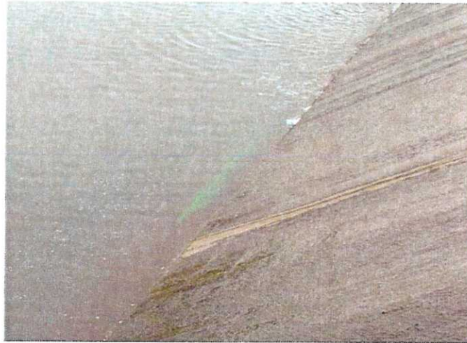
Photo 6 – March 2005, Midco Diving dye testing reveals a small plume of dye at the base of the spillway face prior to the dye flowing over the spillway.
