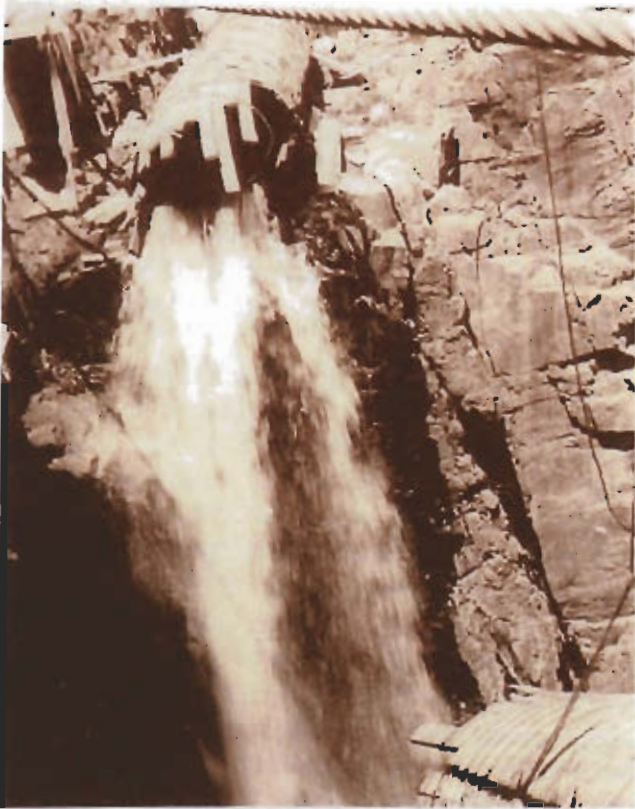
A common problem with the flume was leaks and damage because of weather or weak construction.
