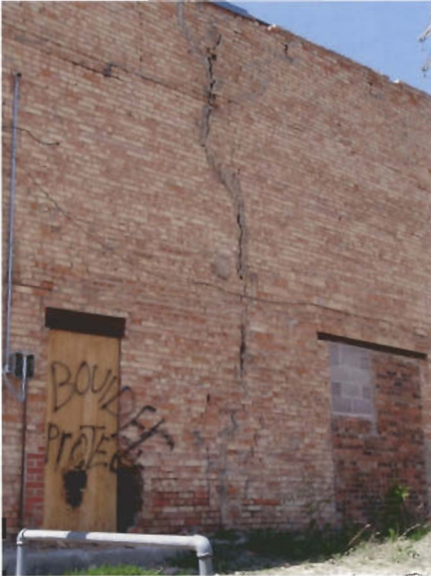
EAST WALL WITH CRACK
